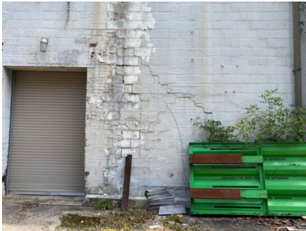
Sagging grade beam & cracked masonry at west side
