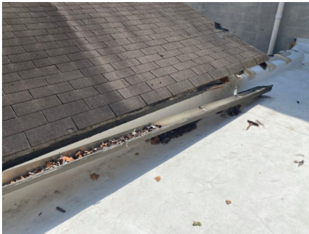
Damaged gutter at east side
