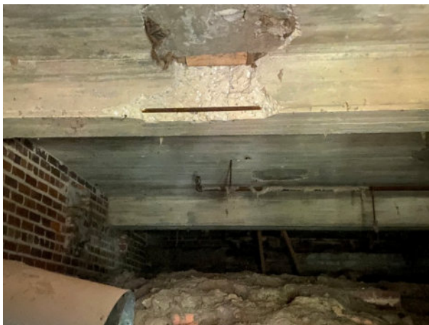
Damaged concrete beam in crawlspace
