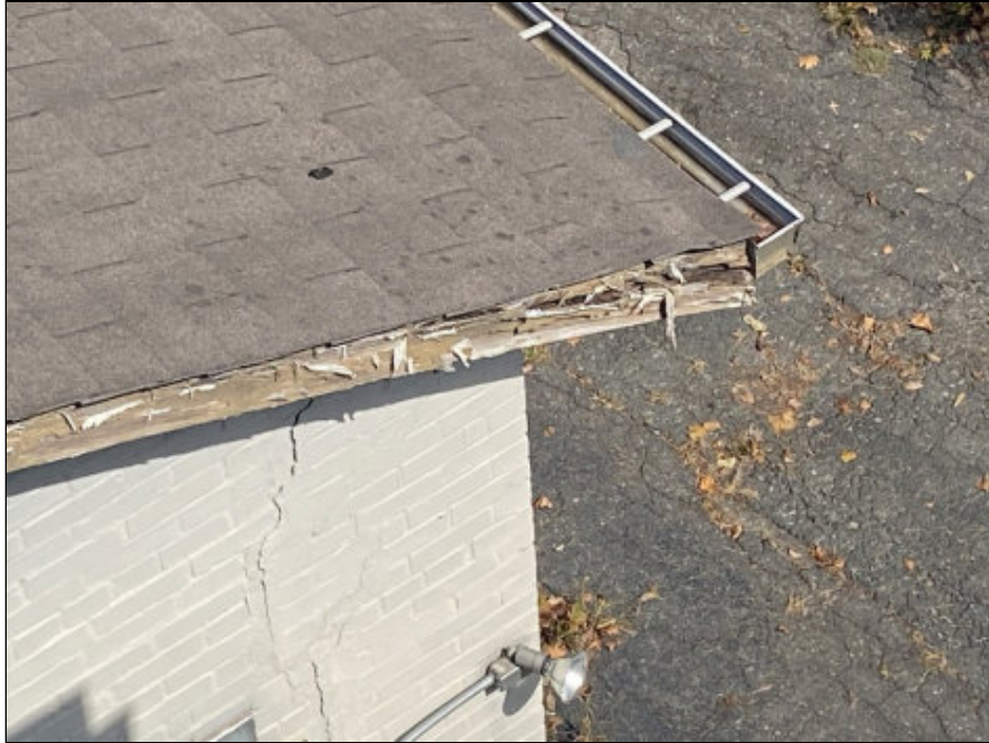
51 - Damaged wood fascia at east side
