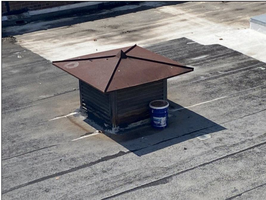
72 - Exhaust vent at west wing
