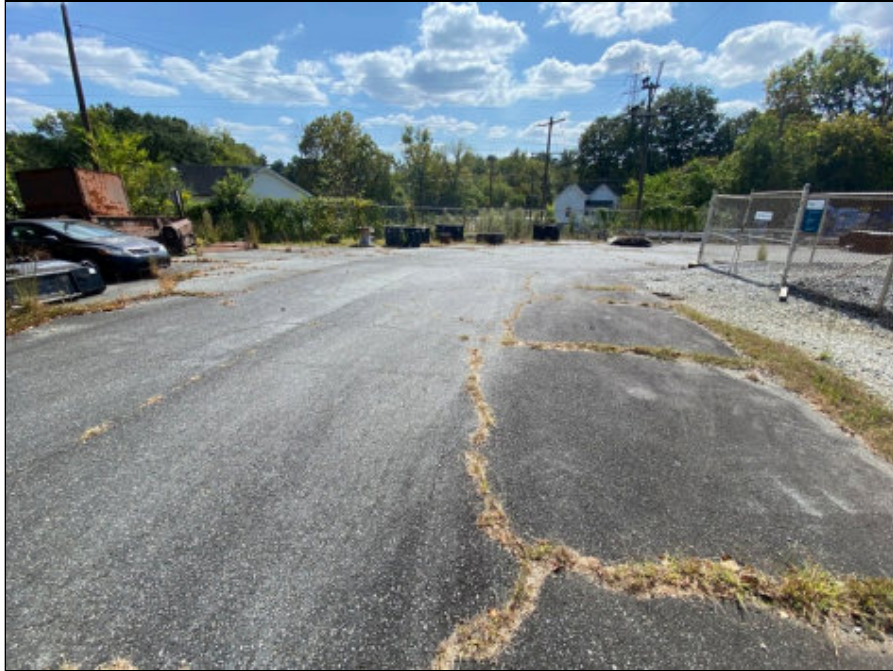
23 - Deteriorated asphalt paving at east side
