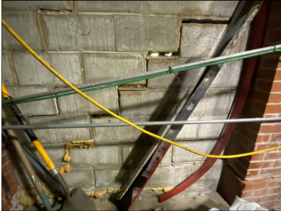
33 - Cracked masonry at west side (interior view)
