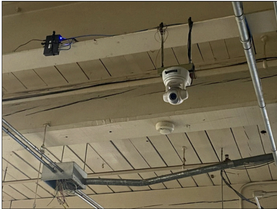
118 - Typical security system camera
