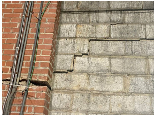
Cracked masonry at west side (interior view)
