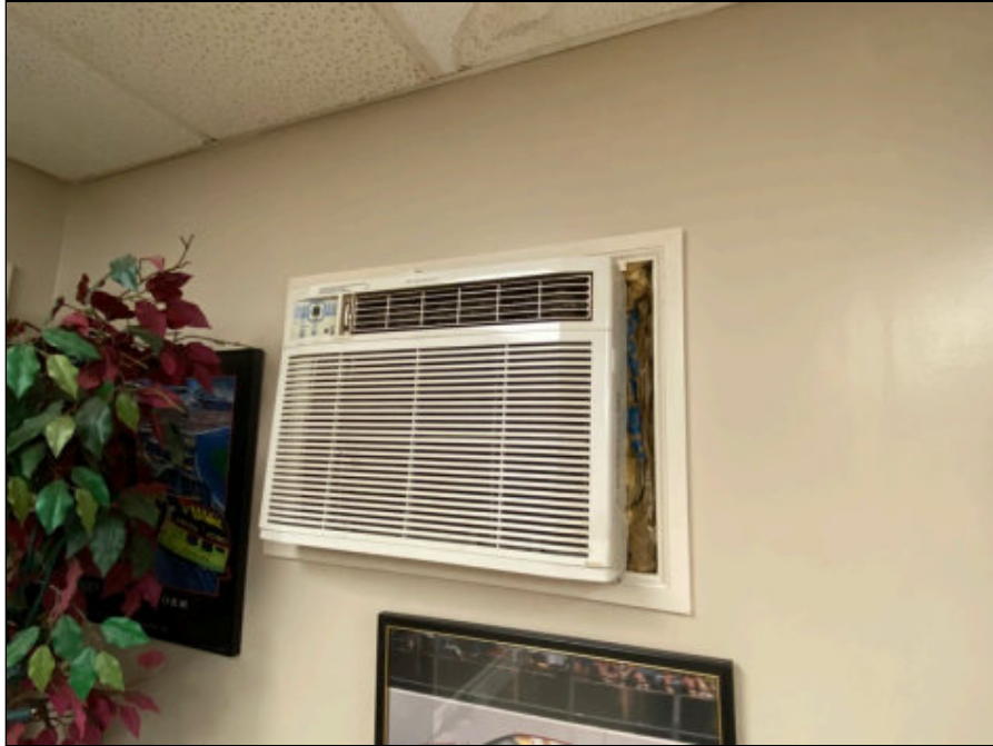
85 - Typical window air conditioner
