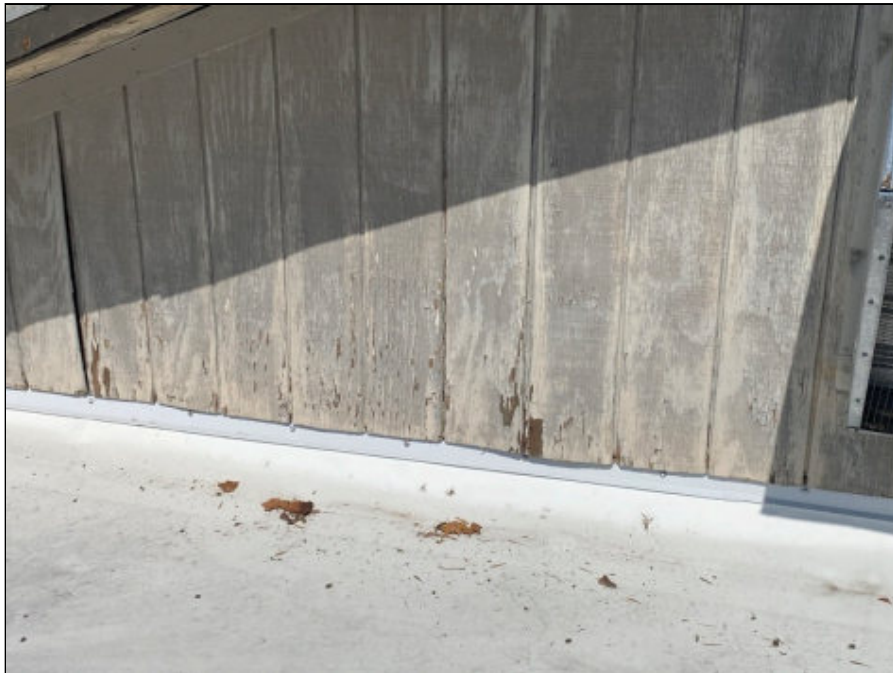
50 - Failed paint on penthouse
