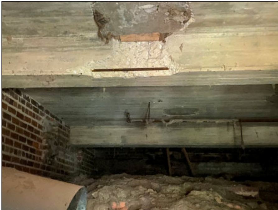
40 - Damaged concrete beam in crawlspace
