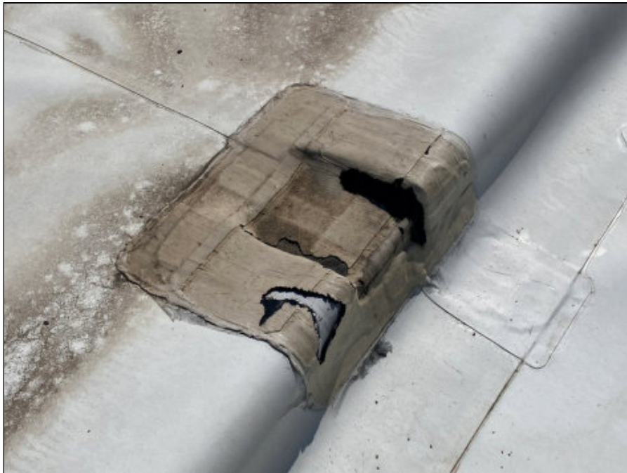
74 - Deteriorated patch at main roof
