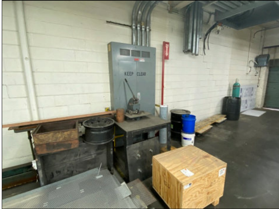
95 - Blocked electrical panel
