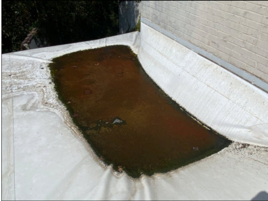
69 - Ponding near elevator penthouse
