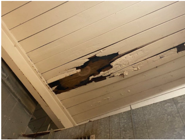
Deteriorated wood roof decking
