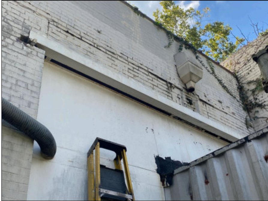
45 - Cracked masonry at west side
