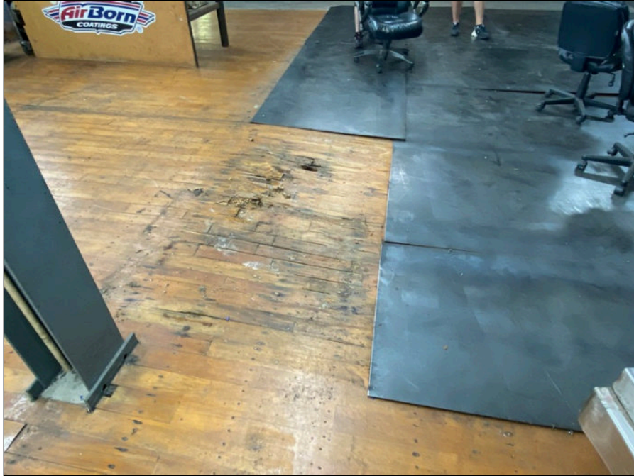
141 - Sagging floor in plant area
