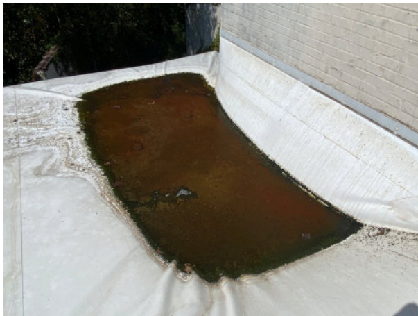
Ponding near elevator penthouse
