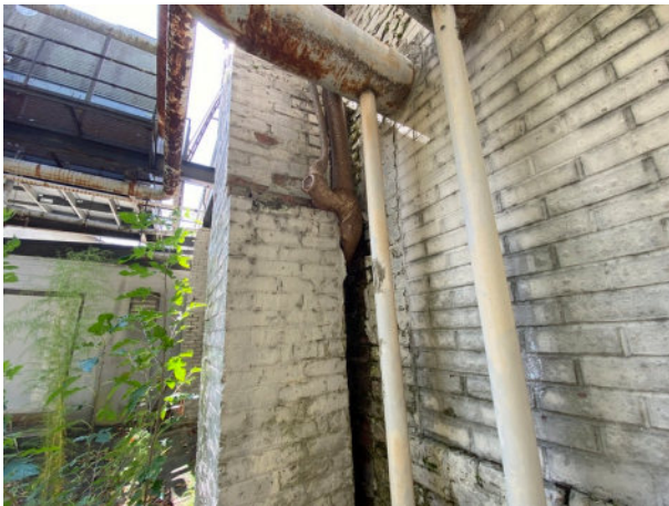
Damaged masonry pier at east side (note tree in pier)
