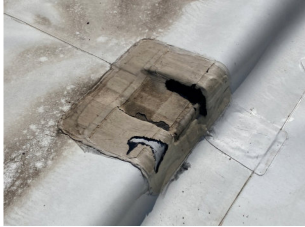
Deteriorated patch at main roof
