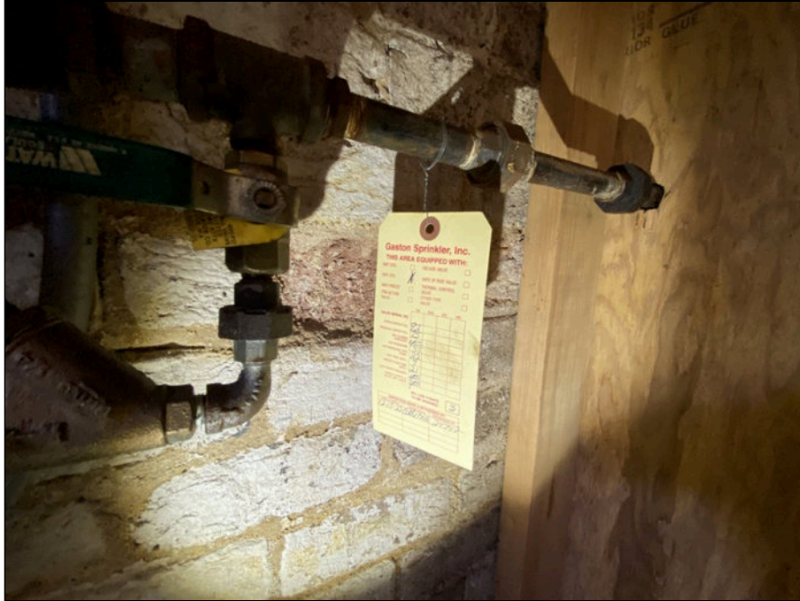
107 - Typical dry sprinkler inspection tag
