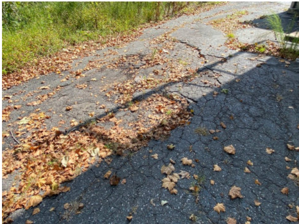
Deteriorated asphalt paving at east side
