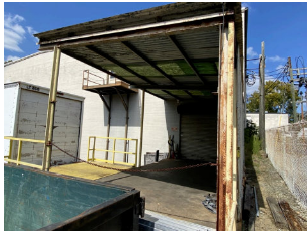
Corrosion at loading dock canopy framing
