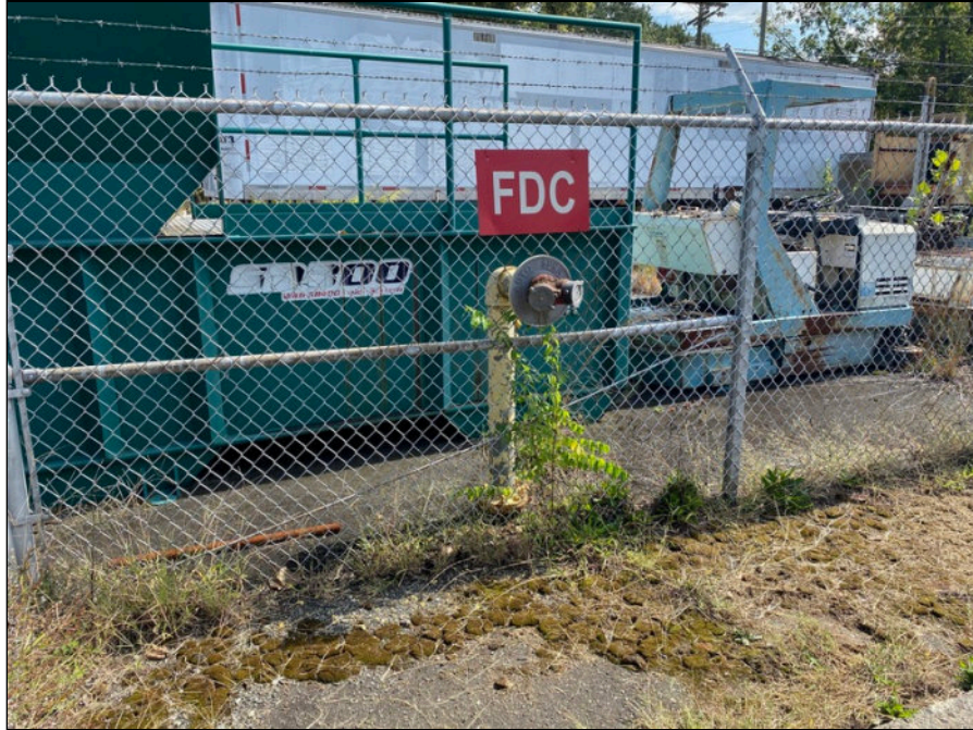
109 - Fire department connection (FDC)
