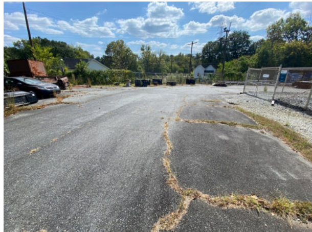
Deteriorated asphalt paving at east side
