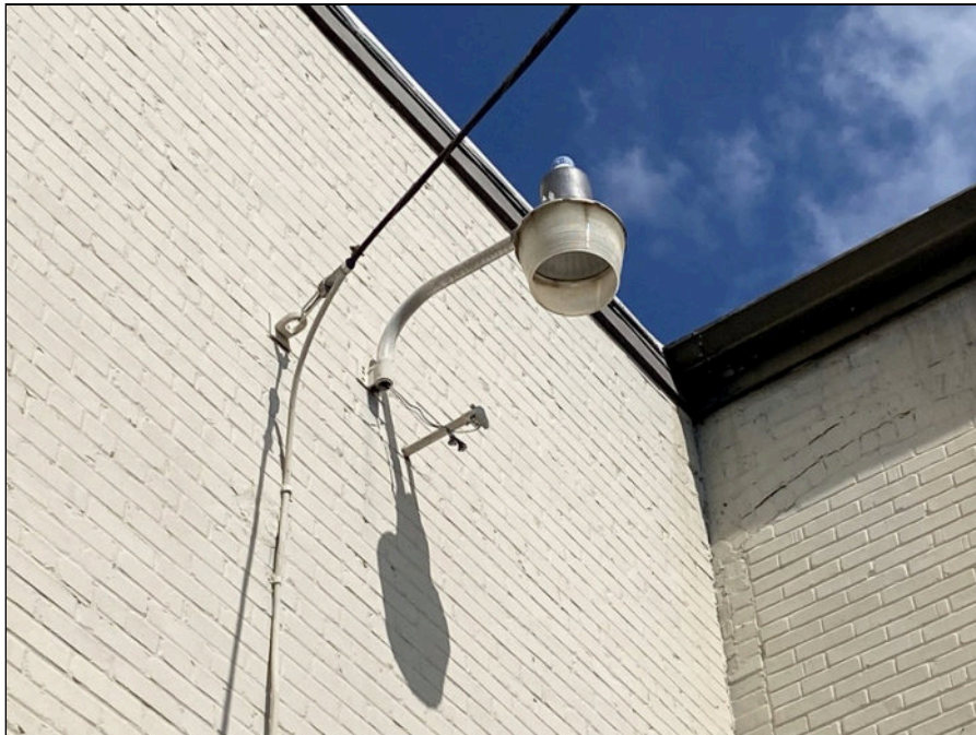
26 - Typical building-mounted light fixture
