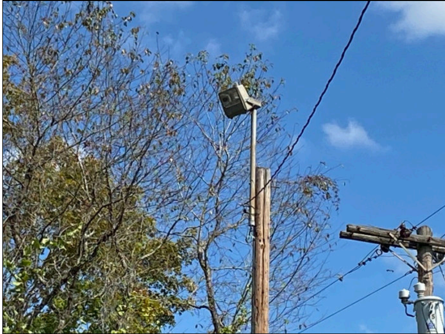
25 - Typical pole-mounted light fixture
