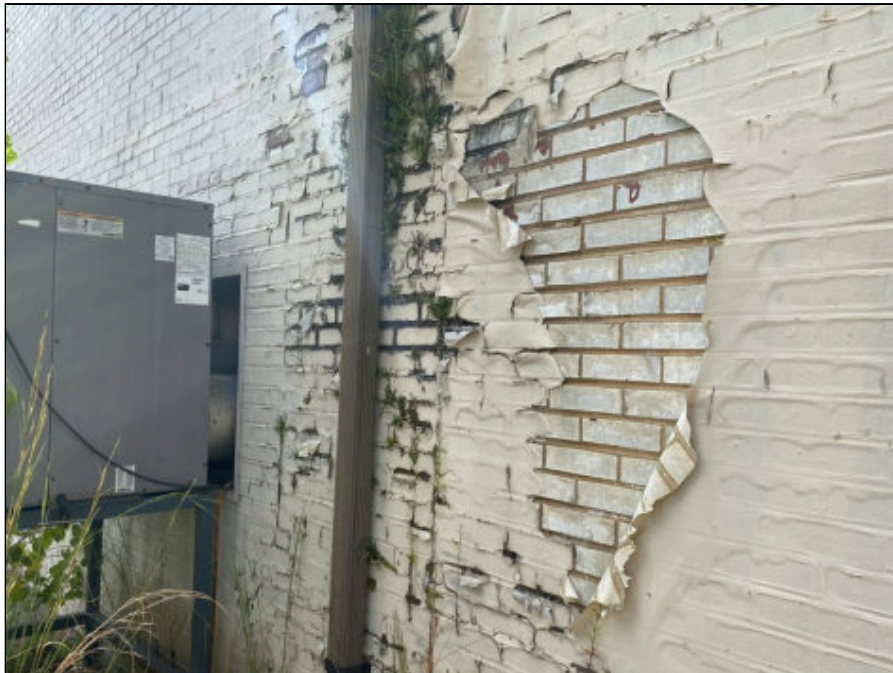
44 - Failed paint on masonry
