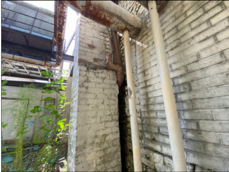
43 - Damaged masonry pier at east side (note tree in pier)
