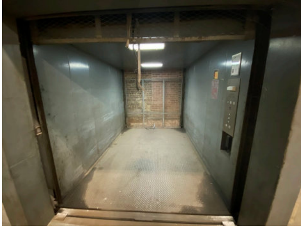
Freight elevator cab
