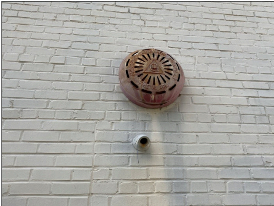
112 - Typical sprinkler alarm bell
