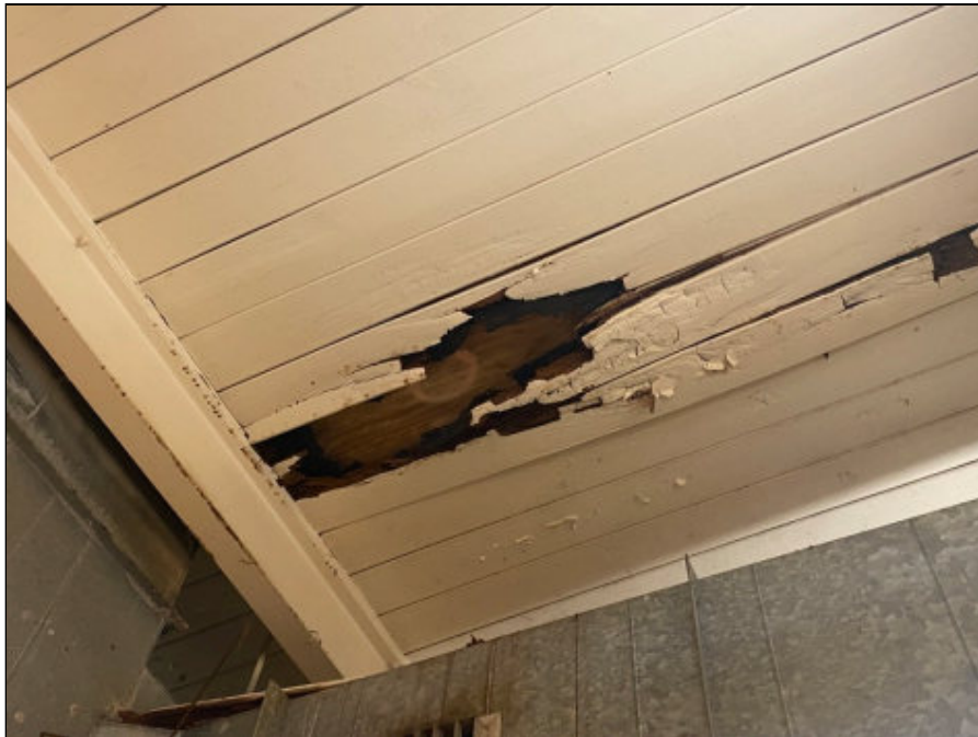
36 - Deteriorated wood roof decking
