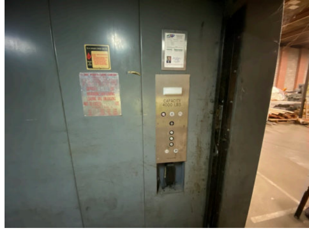
Freight elevator controls
