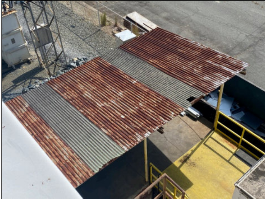
79 - Corroded metal roofing at loading area
