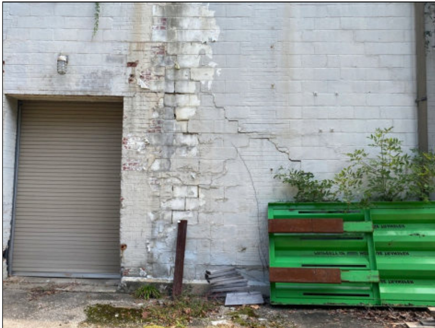
30 - Sagging grade beam & cracked masonry at west side
