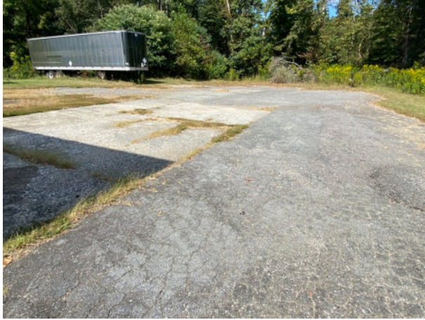
Deteriorated asphalt & concrete paving at north end
