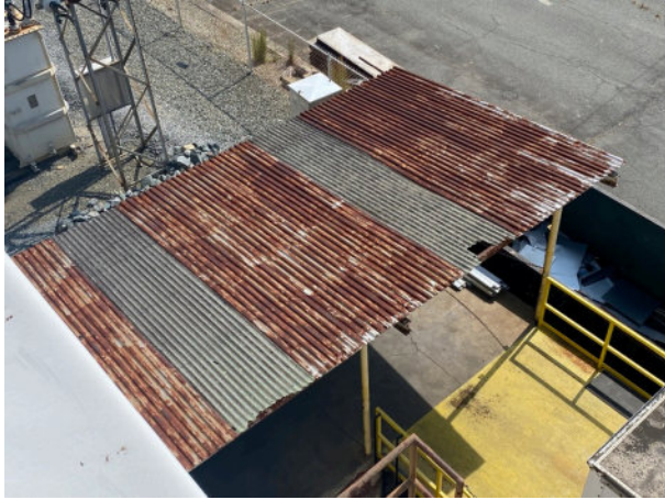
Corroded metal roofing at loading area
