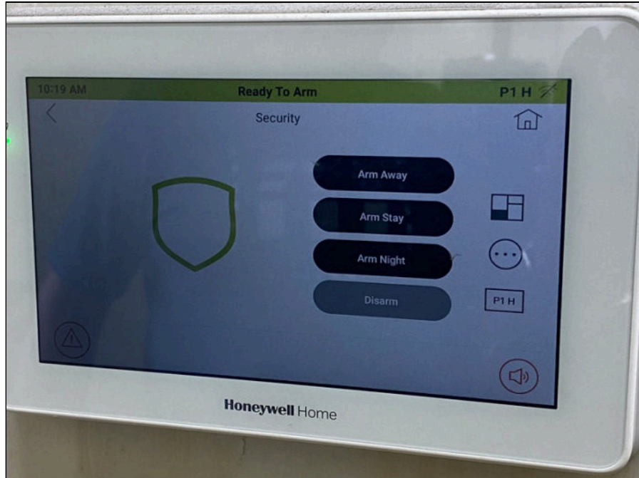
117 - Security system control panel
