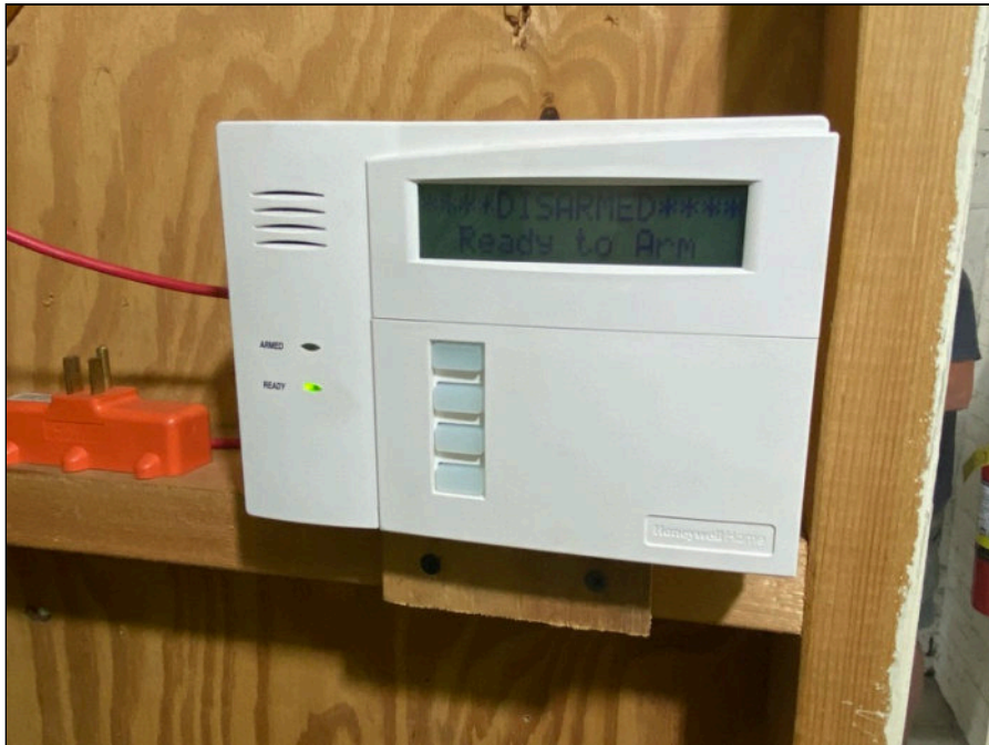
116 - Security system control panel
