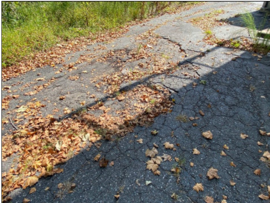
22 - Deteriorated asphalt paving at east side
