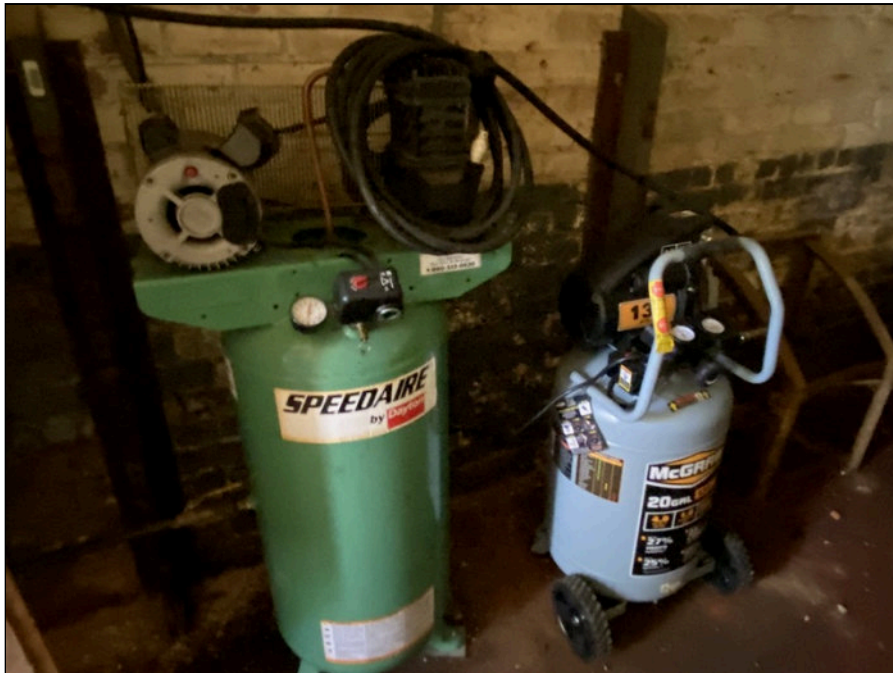
106 - Compressor for dry sprinkler system
