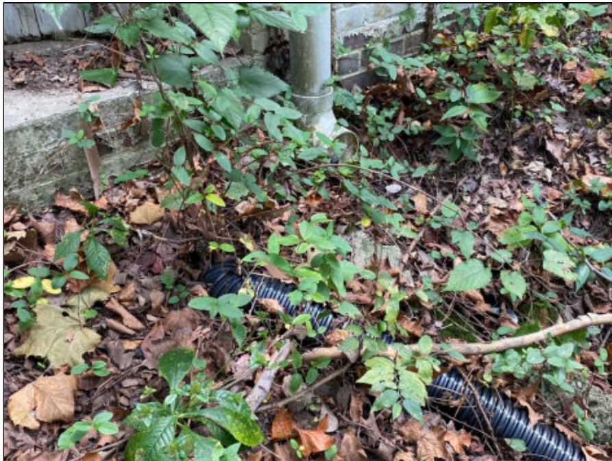
78 - Detached drain line at downspout (west side)
