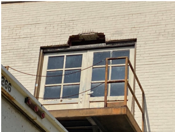
Damaged masonry at door head
