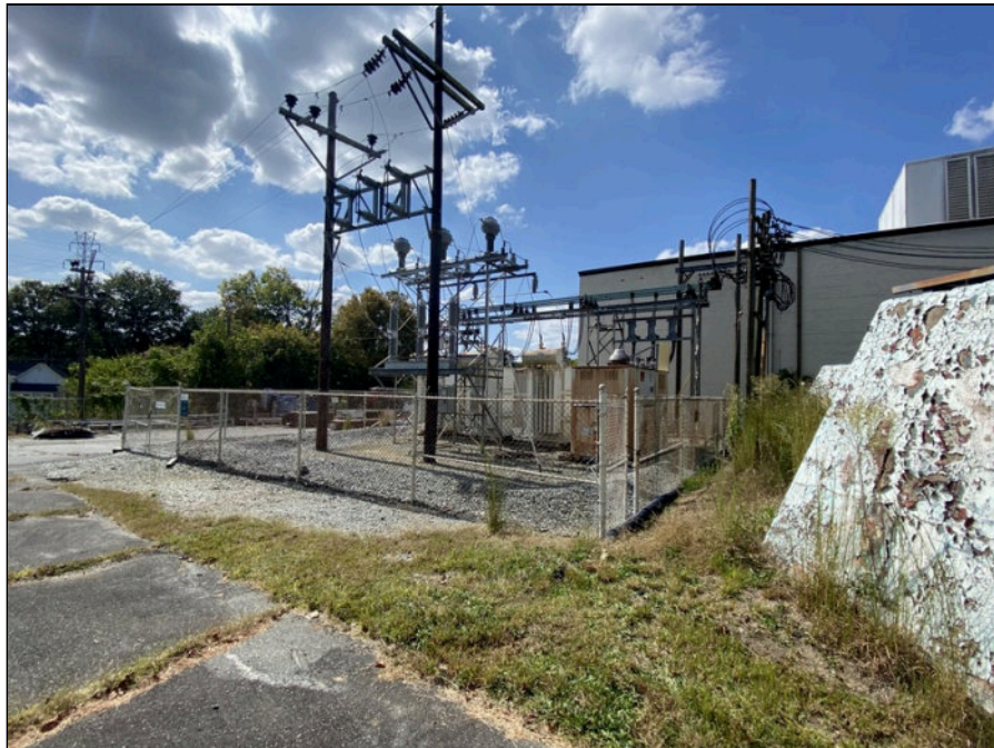
90 - View of electrical substation at east side
