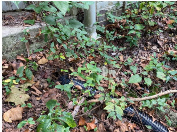
Detached drain line at downspout (west side)
