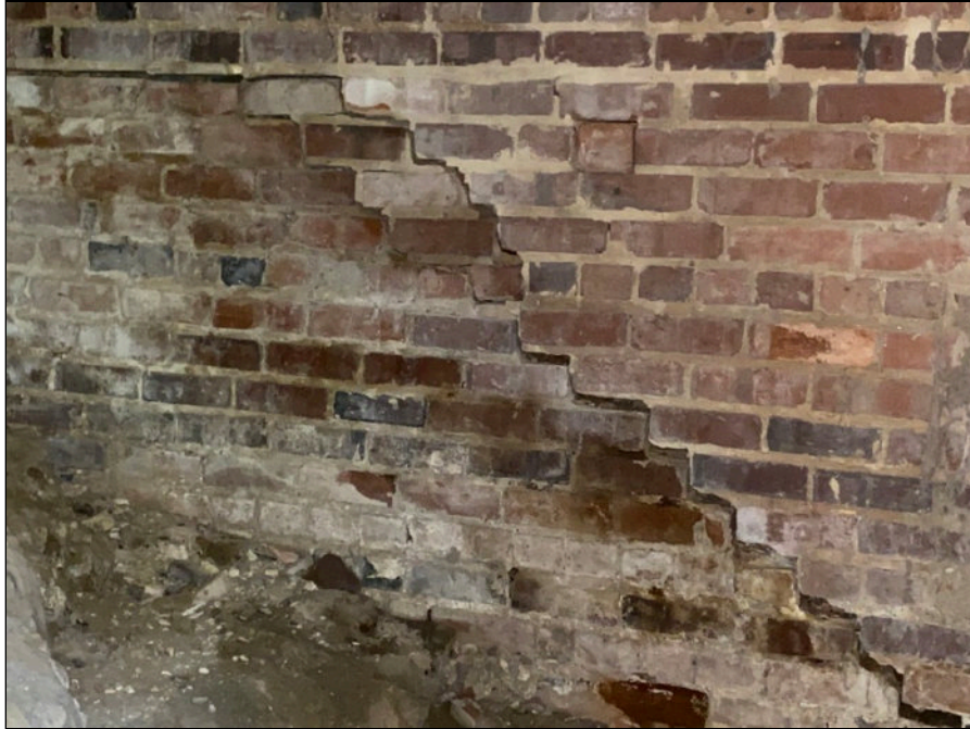
41 - Cracked masonry in crawlspace
