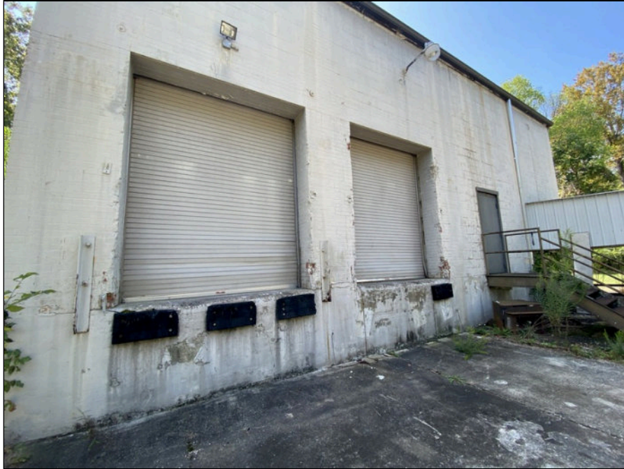
55 - Typical overhead doors
