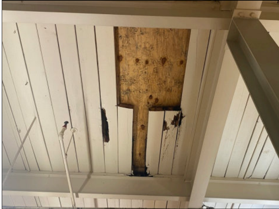
37 - Poorly-supported plywood at gap in roof deck
