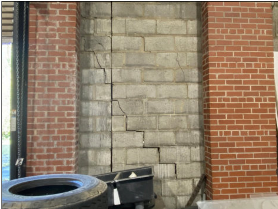
32 - Cracked masonry at west side (interior view)
