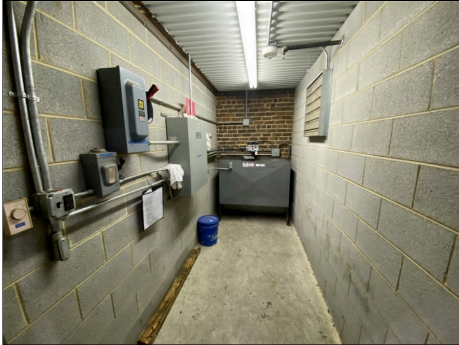
99 - Elevator machine room
