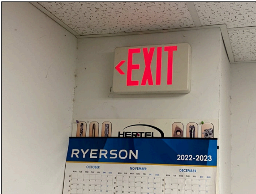
114 - Typical exit sign
