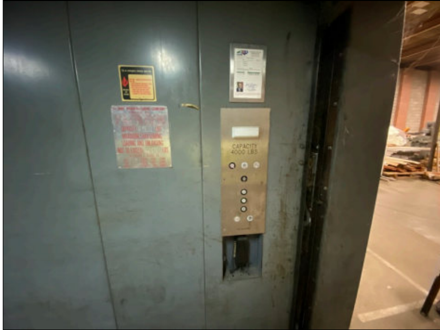
97 - Freight elevator controls
