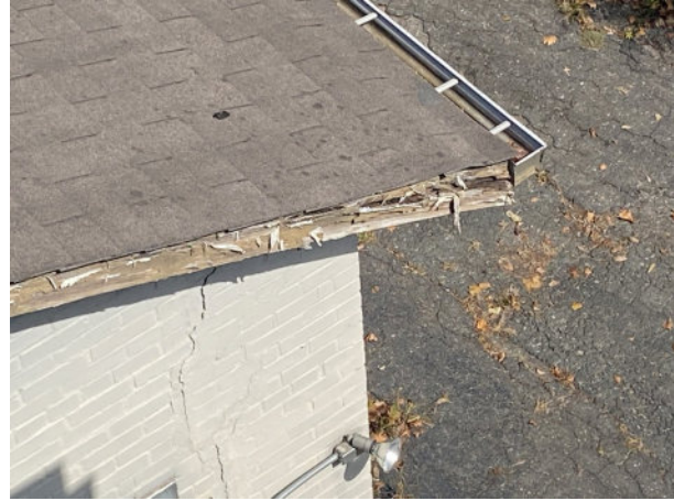
Damaged wood fascia at east side
