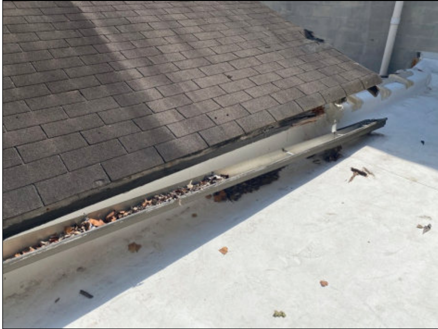
77 - Damaged gutter at east side
