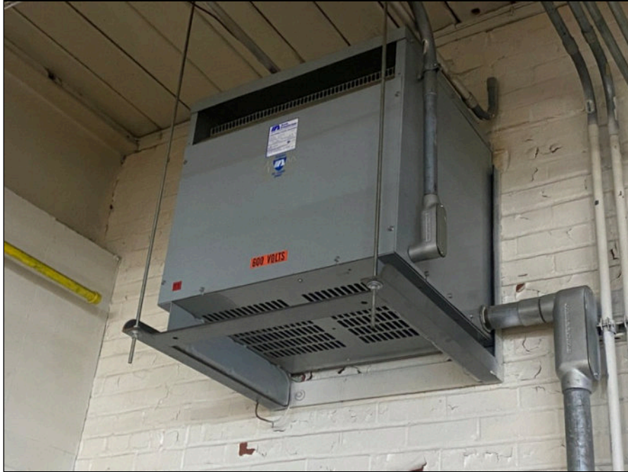
93 - Typical step-down transformer
