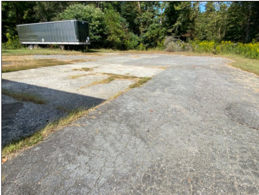
24 - Deteriorated asphalt & concrete paving at north end
