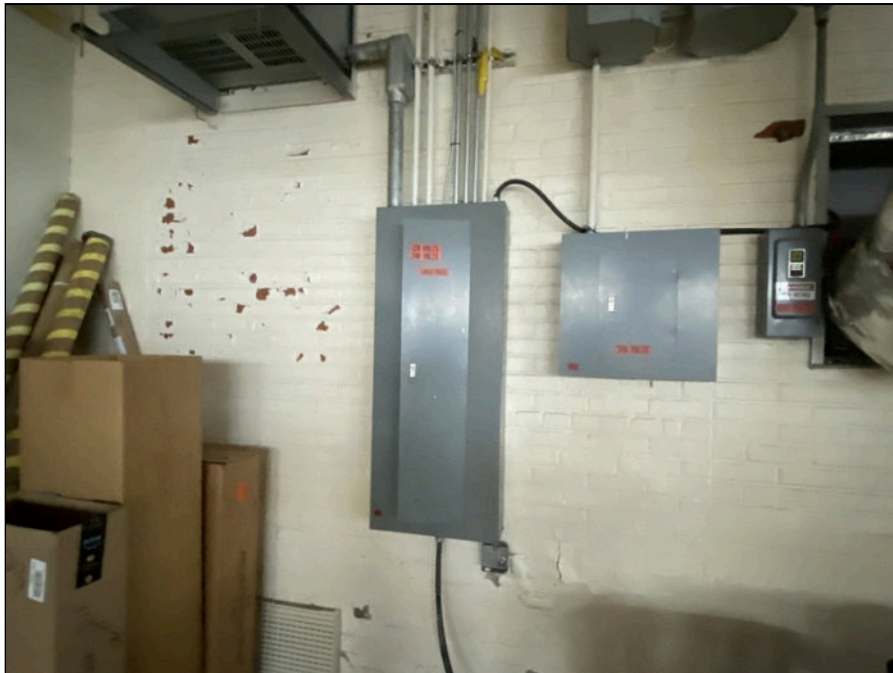
94 - Typical electrical panel
