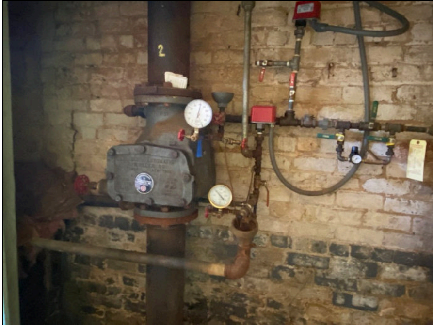
105 - Typical dry sprinkler riser
