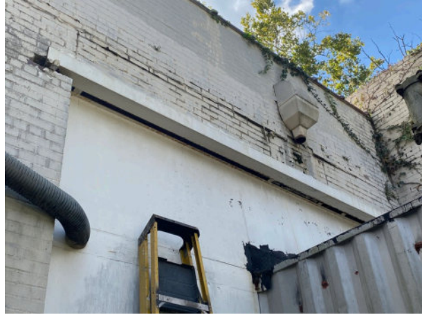
Cracked masonry at west side
