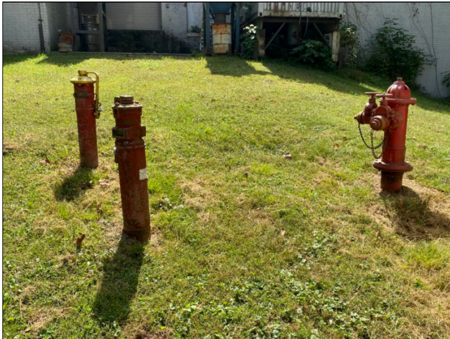
108 - Typical hydrant & PIVs
