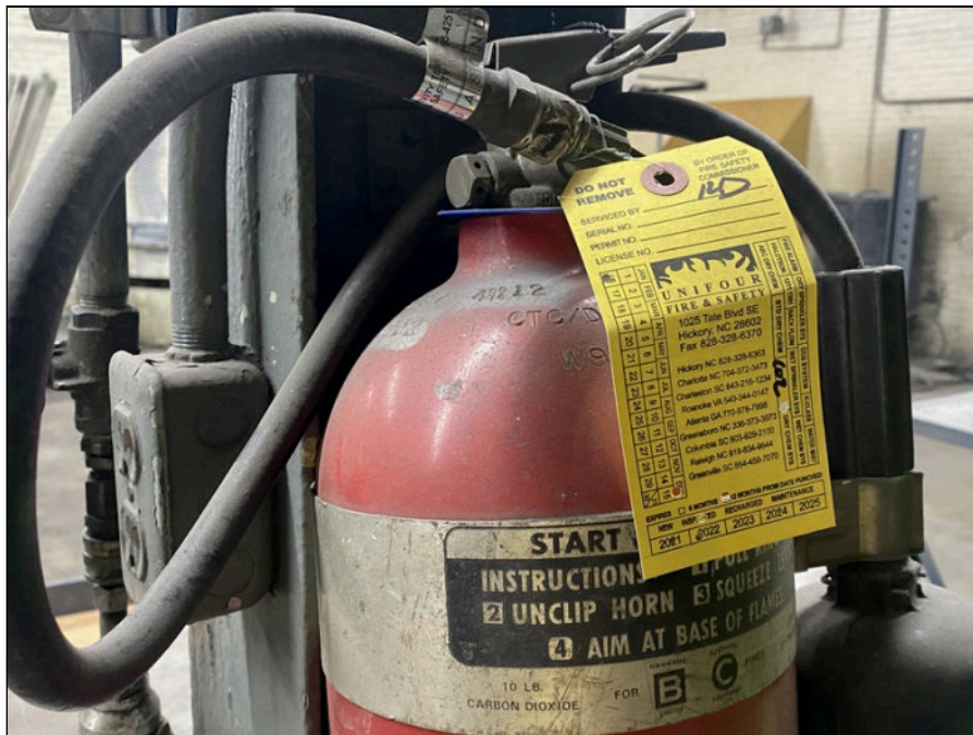
110 - Typical CO2 fire extinguisher
