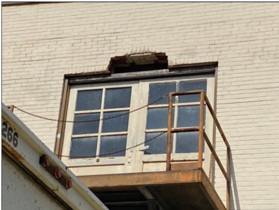
48 - Damaged masonry at door head
