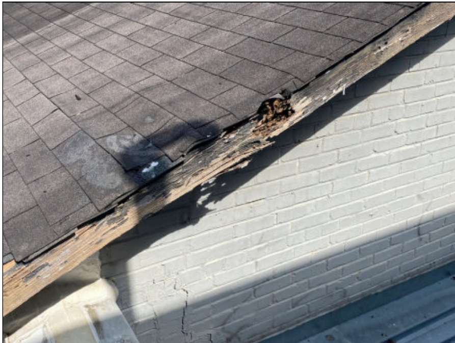
52 - Damaged wood fascia at east side
