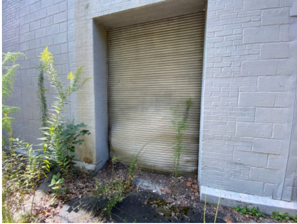
Damaged overhead door
