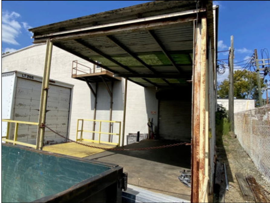
49 - Corrosion at loading dock canopy framing
