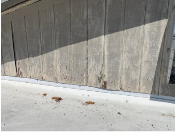
Failed paint on penthouse
