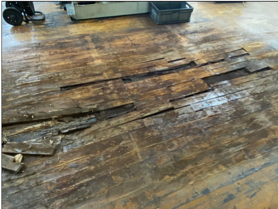
140 - Damaged flooring in plant area
