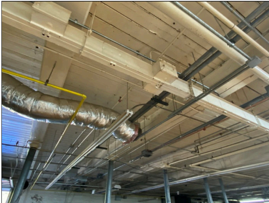
92 - Electrical bus duct (at center)
