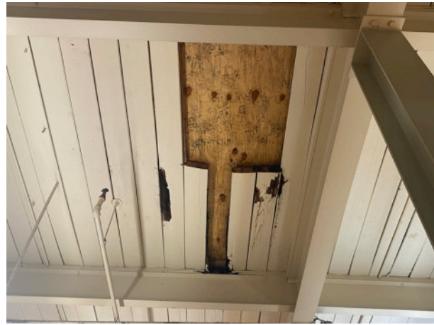
Poorly-supported plywood at gap in roof deck
