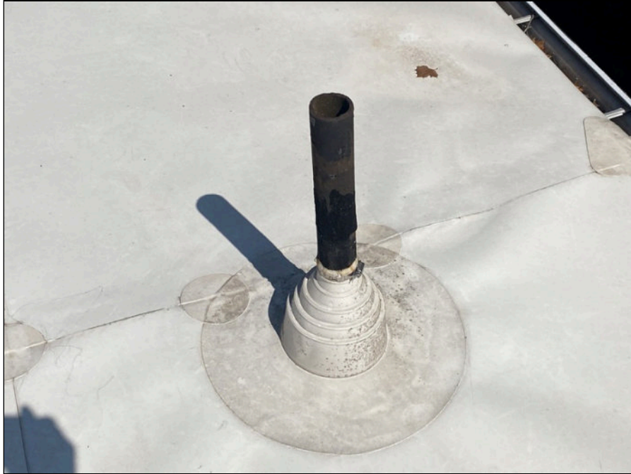
67 - Typical vent pipe
