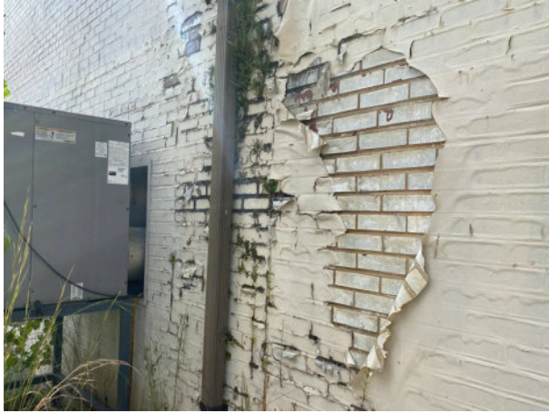
Failed paint on masonry
