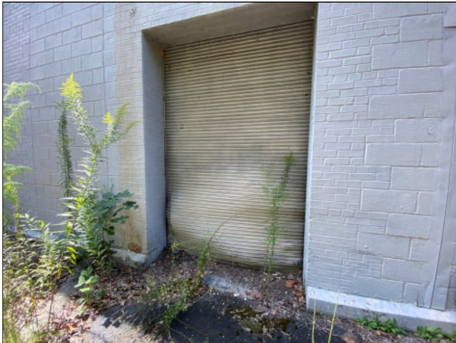
56 - Damaged overhead door
