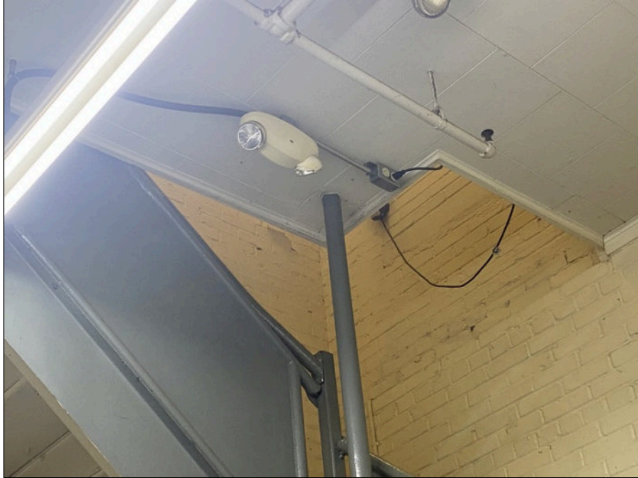
115 - Typical emergency lights
