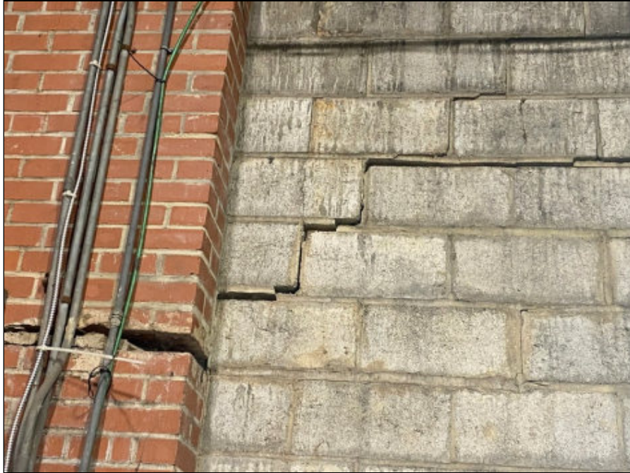
31 - Cracked masonry at west side (interior view)
